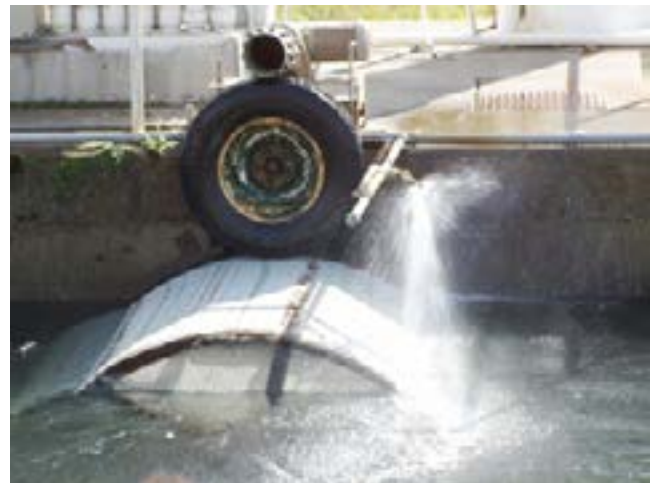
Outer cleaning jets spraying debris off
