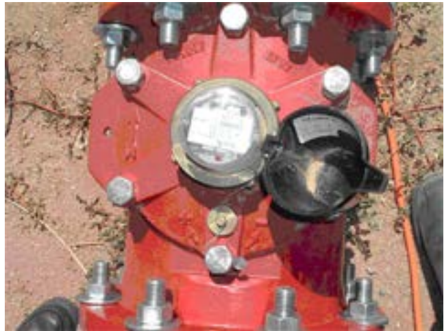
Figure 7-46 Typical in-line recording flowmeter
