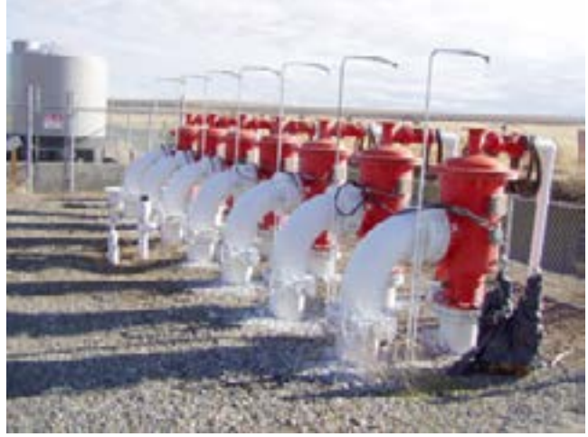
Figure 7-29 A battery of automatic flushing screen filters
