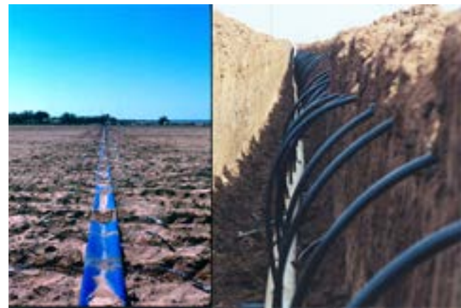
Layflat flexible manifold on the surface and a buried rigid PVC manifold
