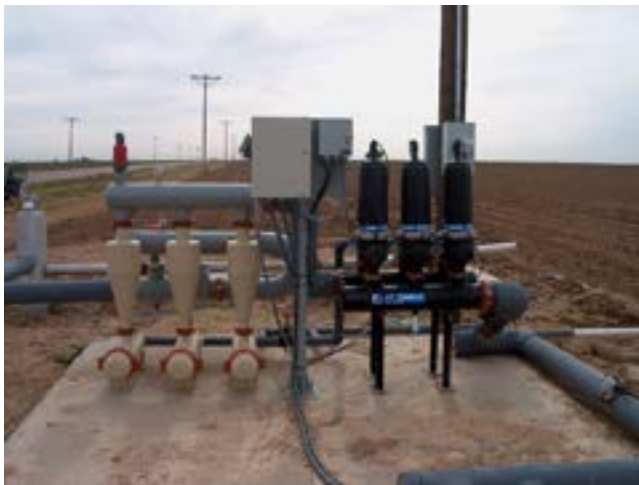
Figure 7–36 A three-unit vortex sand separator system (to the left of disk filters)
