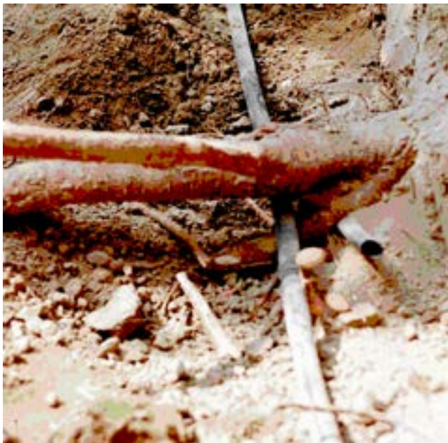
Figure 7–13 An example of a root pinching the SDI lateral (cut lateral on the right) in a pistachio orchard with the SDI lateral installed 5 feet (1.52 m) from the tree row and 18 to 20 inches (0.46–0.51 m) deep
