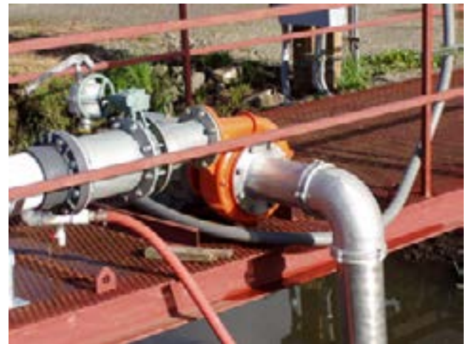
Figure 7–21 Pumping station using a low head centrifugal pump
