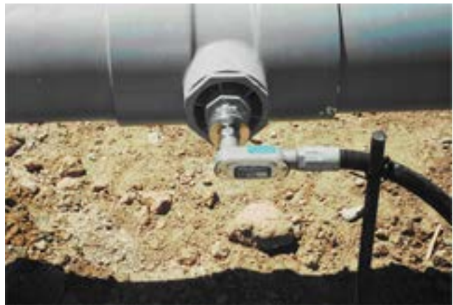
Figure 7-47 Paddle wheel electronic flowmeter installed in a large-diameter mainline
