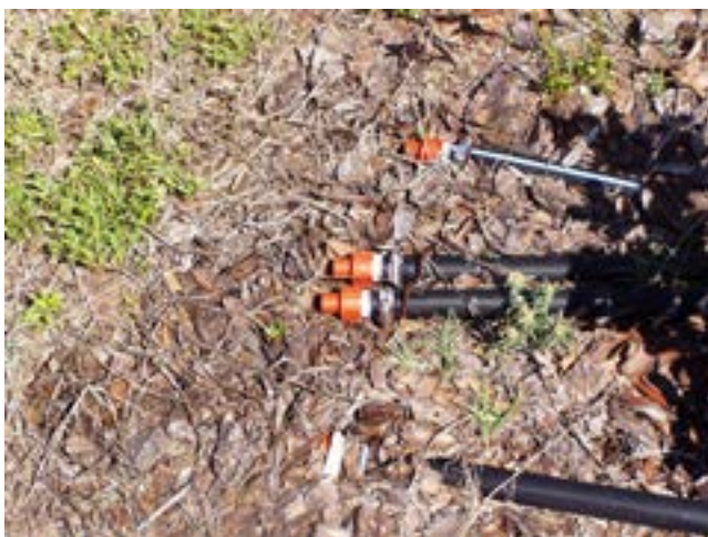
Figure 7-90 Example of end of line flushing valves
