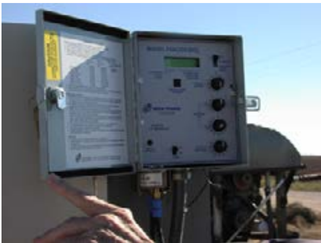
Automated control system panel (courtesy of Jerry Walker)
