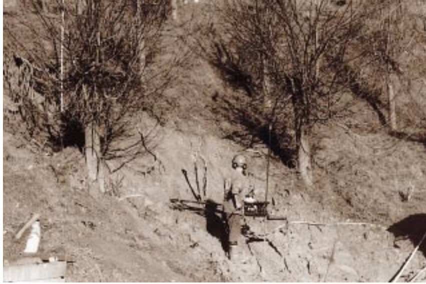
Portable drilling equipment used to install horizontal bore draws. This bore produced an initial flow of approx 3,500L per hour and prevented further slope instability.
