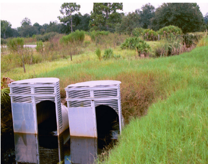
Figure 15. Water control structure used to maintain water level and drainage rate from citrus grove.
