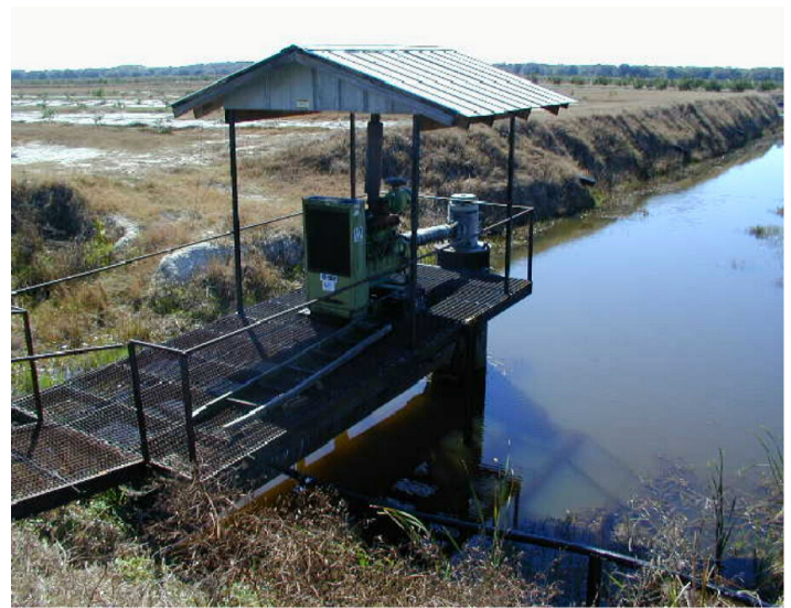
Figure 12. Drainage pump station in citrus grove.
