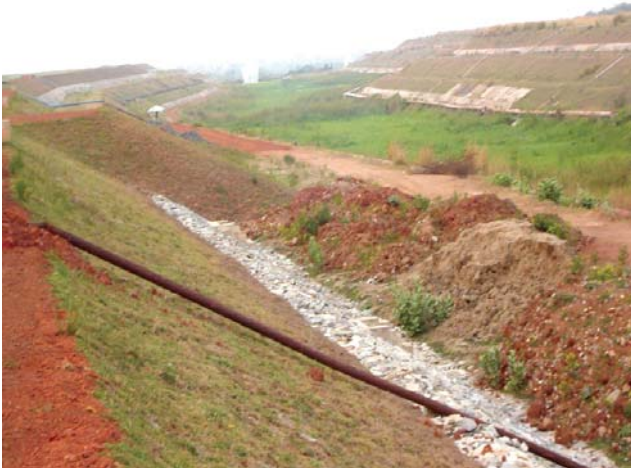
Figure 42. Granite lined canal is discharging ash slurry to wetland
